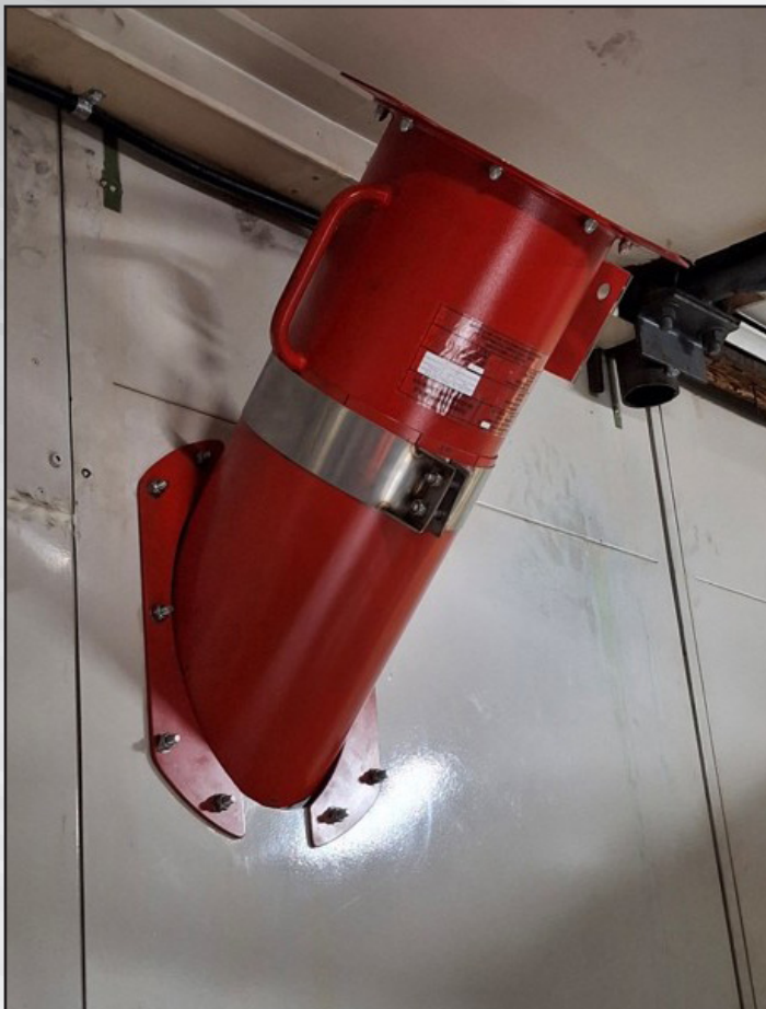
PYROGEN FIRE SUPPRESSION
